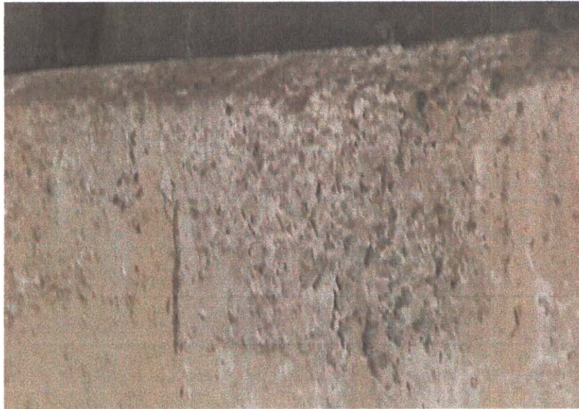
ABUTMENT #1 HONEYCOMBING ON CAP
