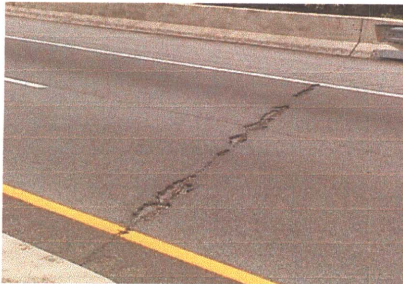
POTHOLE @ JOINT B-APPR-TYPICAL
