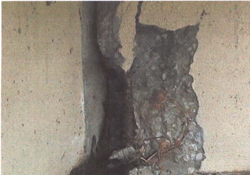
ABUTMENT #1 BREAKOUT WITH EXPOSED REBAR LEFT SIDE
